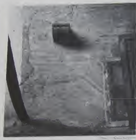
Fig. 301. S. Sustina. South wall of nave, elevations between tenth and eleventh courses, from sky level, side of church.
